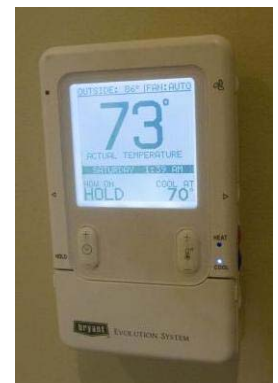
A control panel at the Echelon house in Cherokee County displays the temperature and other information for the homeowner.
