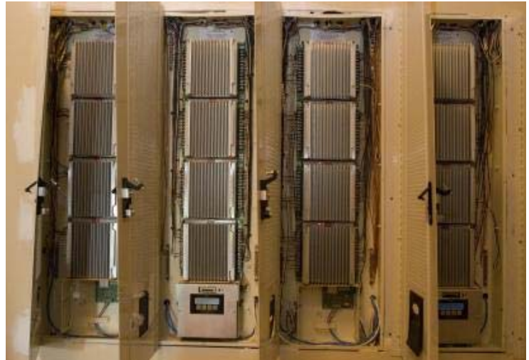
A master control panel in Echelon centralizes connections for miles of wiring.
