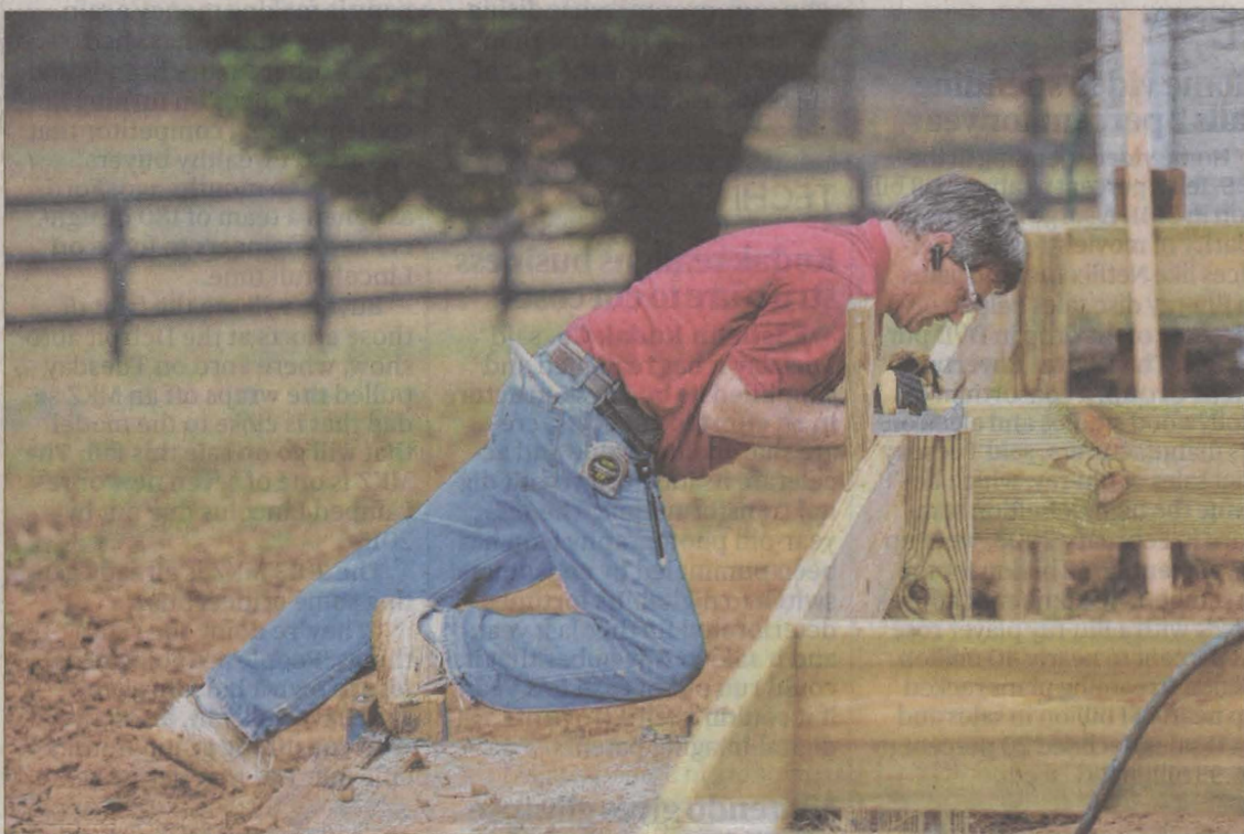
Builder Tony Pourhassan works on a deck Tuesday in Sharpsburg. He founded the Georgia Redevelopment Foundation to help homeowners keep up home maintenance. Johnny Crawford jrcrawford@ajc.com
