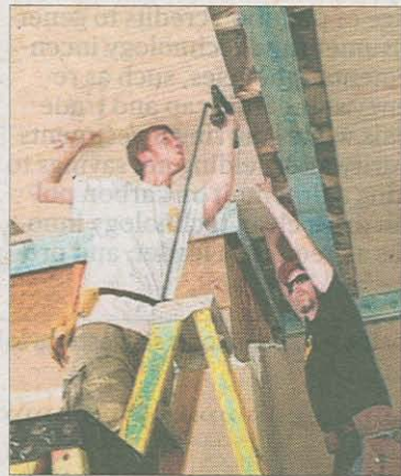
Atlanta Design & Build Project Manager David Newell (right) and apprentice Courtney Olson work on a home recently in Roswell.
